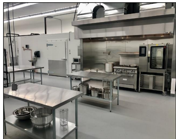
Figure 4: SKRFH Kitchen (SKRFH, n.d.)
