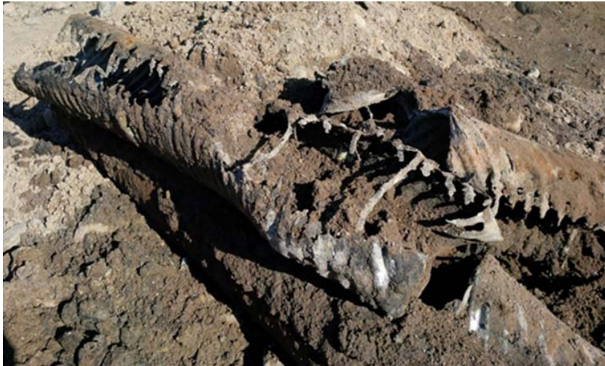
Photo: Failed CMP sewer main showing no bottom left in the pipe.
