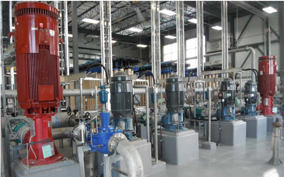
Photo: View of water supply pumps on the main floor, with beige filtration racks in the background.
