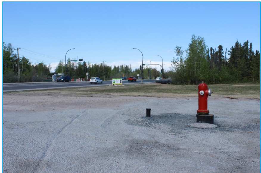
This new fire hydrant next to the station allows firefighters to train without compromising response times. City of Yellowknife Photo.
