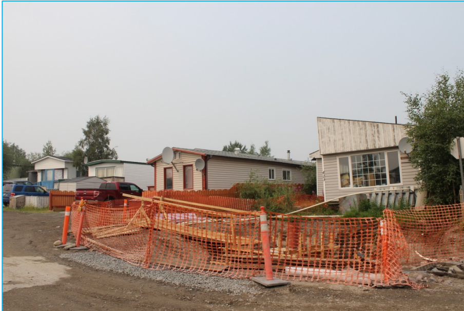
Properties in Northland undergoing water and sewer replacement. City of Yellowknife photo.
