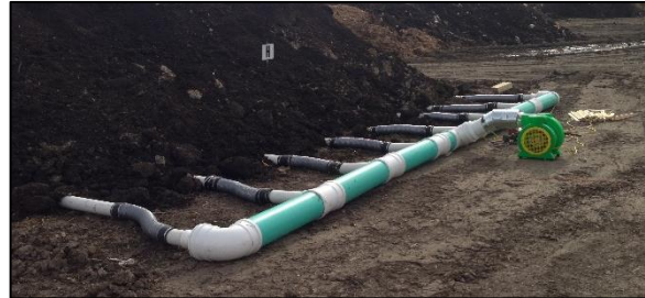
FIGURE 1 ASP SYSTEM AT STICKLAND FARMS (PENHOLD, AB)
