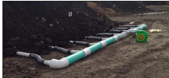
Figure 77 : ASP System at Stickland Farms (Penhold, AB)
