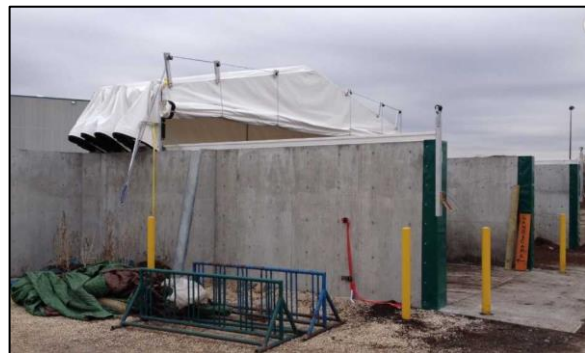
FIGURE 6 AGGREGATE BUNKER WITH ROLLCOV-R ROOF SYSTEM (SOURCE: CHAMELEON INNOVATIONS)
