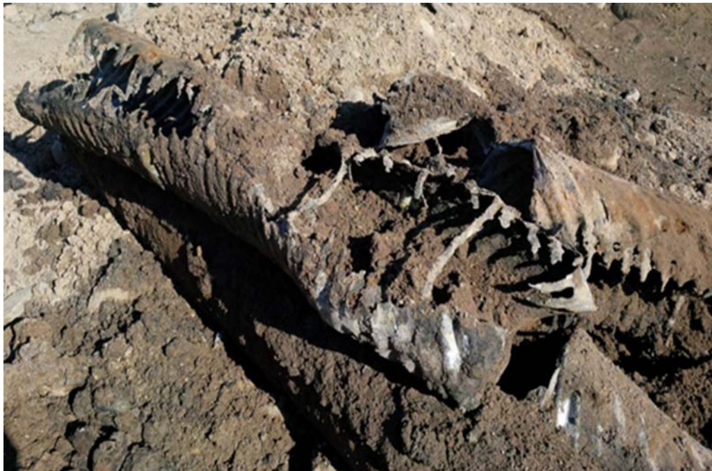
Photo: Failed CMP sewer main showing no bottom left in the pipe
