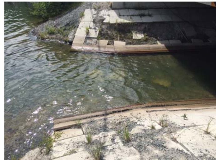
Photo: Showing erosion control methods failing causing abutment destabilization.
