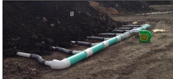
Figure 77 : ASP System at Stickland Farms (Penhold, AB)
