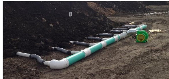
FIGURE 1 ASP SYSTEM AT STICKLAND FARMS (PENHOLD, AB)
