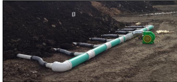
FIGURE 1 ASP SYSTEM AT STICKLAND FARMS (PENHOLD, AB)
