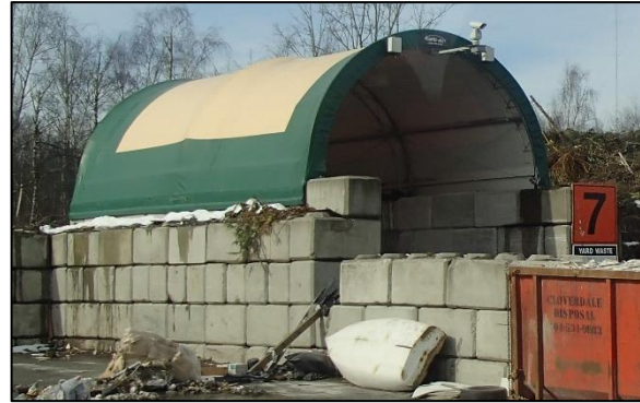
FIGURE 5 ENCLOSED WASTE RECEIVING BUNKER
