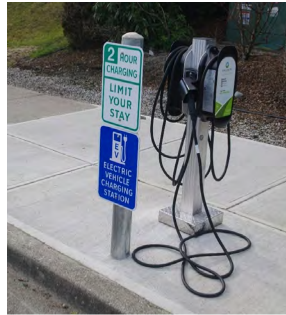
ELECTRIC VEHICLE CHARGING STATION
