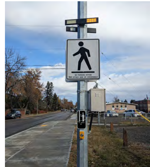
ENHANCED CROSSWALK WITH RECTANGULAR RAPID FLASHING BEACON (RRFB)
