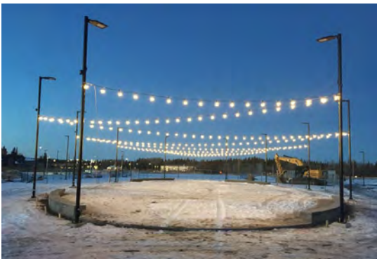
OVERHEAD CATENARY LIGHTING
